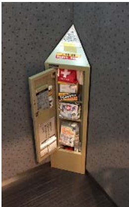
Elevator Emergency Supply Cabinet
