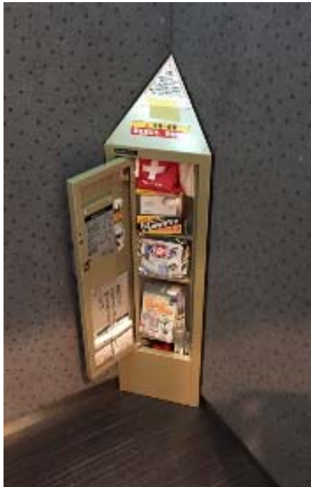
Elevator Emergency Supply Cabinet
